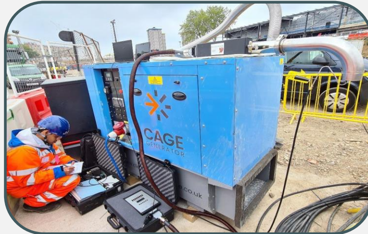
LPG generator at HS2's London, Euston Station
